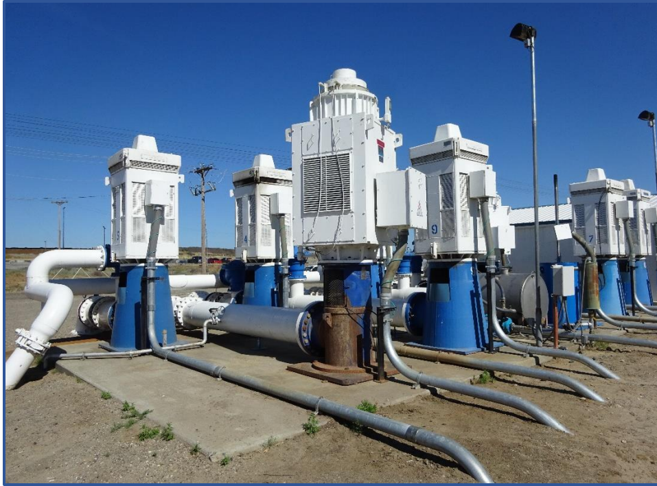
Figure 3. Irrigation Pump Station on Upper McNary Pool, Backwater Area (2022)
