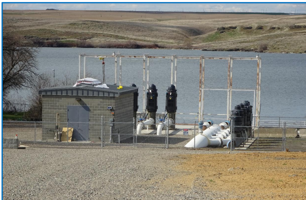
Figure 1. Ice Harbor Pool Irrigation Pump Station, South Shoreline Location (2023)
